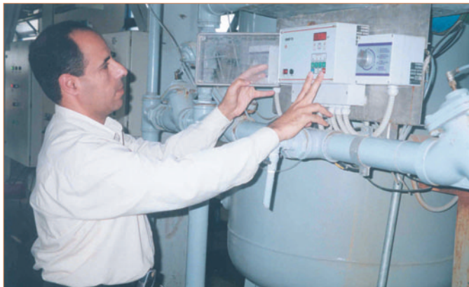
Flue Boiler Tuning
