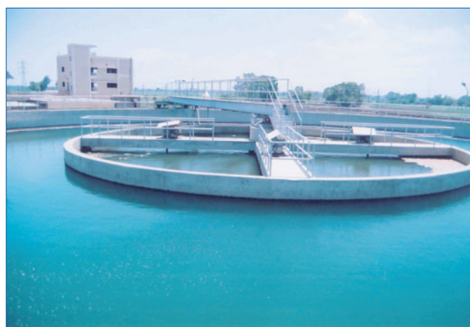
Water Treatment Plant, Bostan Village
