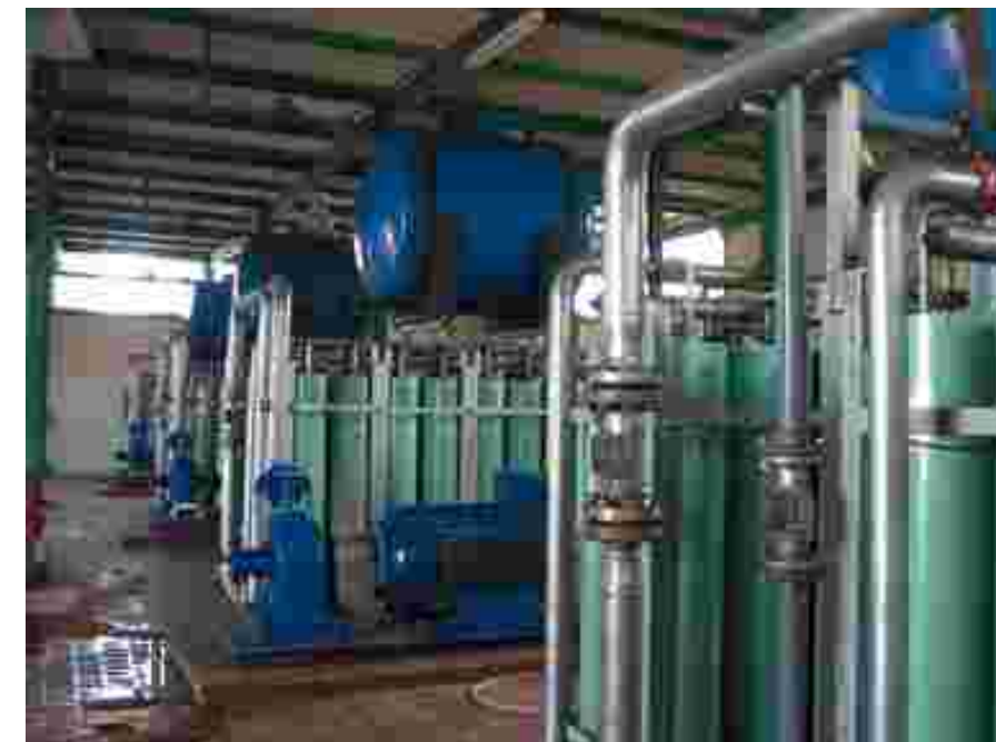
Desalination plant serving Dahab City
