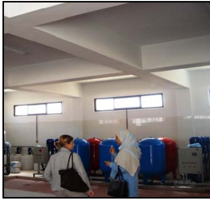
Figure (14) Al-Gefgafah Desalination Plant
