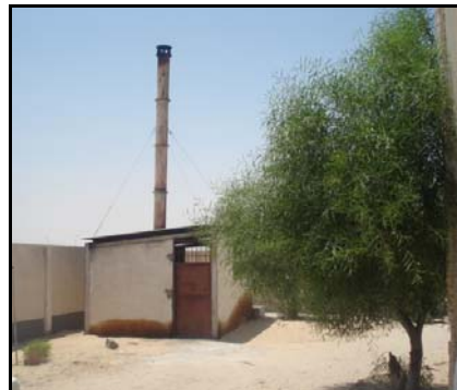
Figure (29) Chest hospital incinerator
