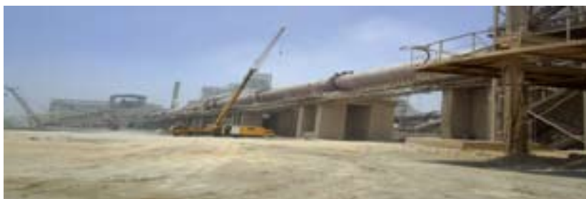
Fig (11-1) Rotary Kiln Line No. (1)
