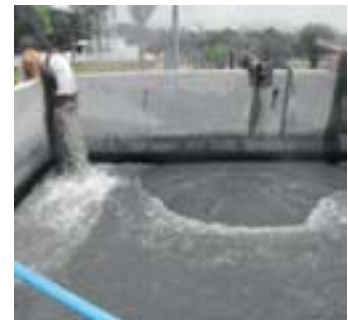
Pic. (5-6) Sewage Wastewater
